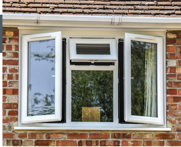
Trickle Vents installed through the window sashes
